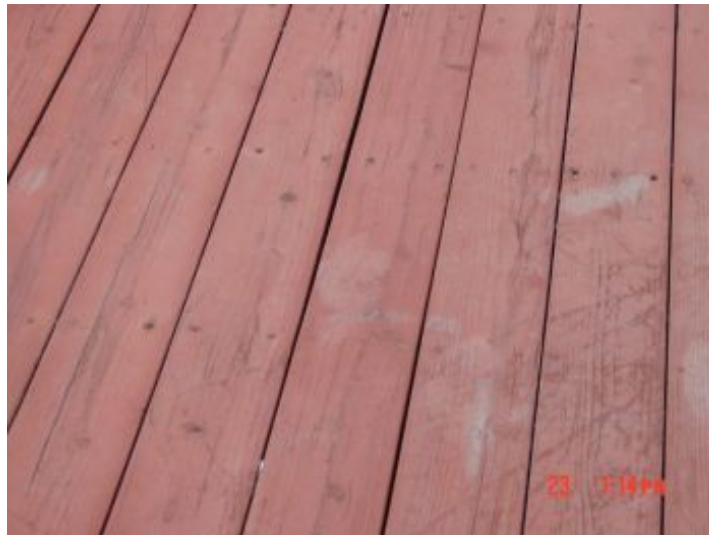
Weathered Deck Boards
